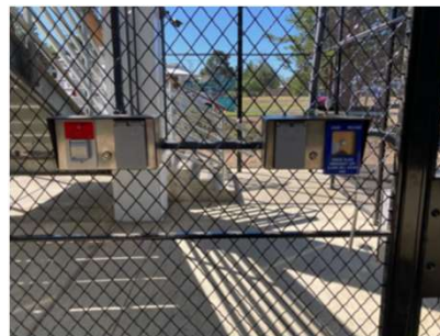
Break Glass to Release Doors
