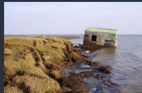
Usteq – permafrost thaw collapse USGS https://dggs.alaska.gov/hazards/permafrost.html
