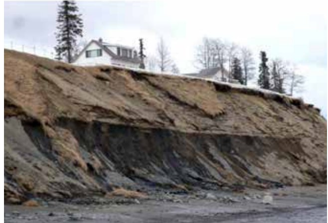
Bluff erosion along Kenai River
